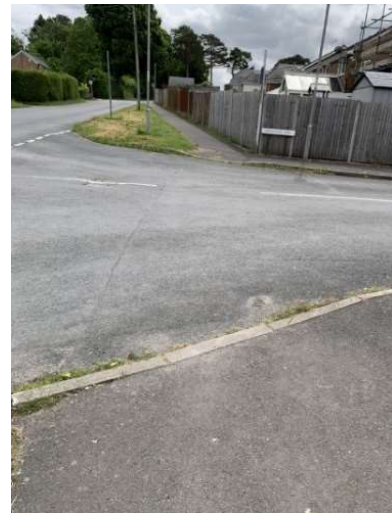
Photograph 14: Crossing infrastructure along Hillbury Road
