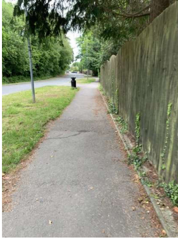
Photograph 1: Footway along Station Road
